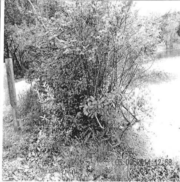
Massive Vegetation on the Upstream Slope of the dam
